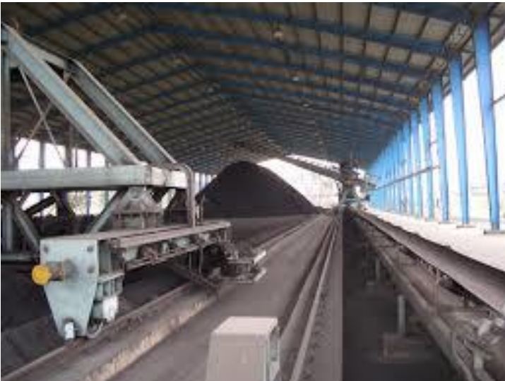
Figure 10.2: Stacker – Reclaimer with covered shed
