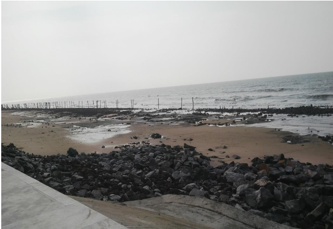
Photo 4.4.10 Seawall at Tajpur in dilapidated condition
